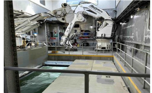
This is the submersible launch area. The crane lifts weight as heavy as a mini-van.
